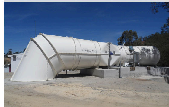
Primary ventilation project in Europe
