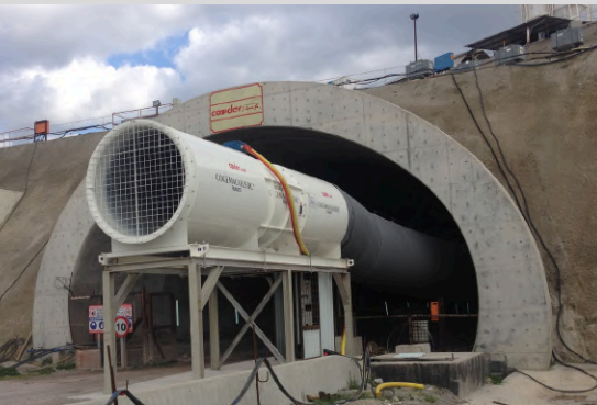
Tunnel ventilation in North Africa
