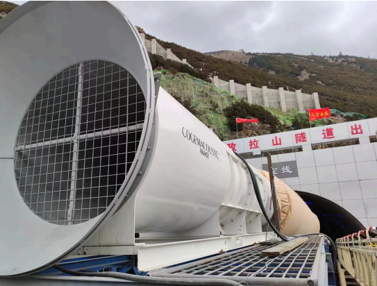
Tunnel ventilation in Asia
